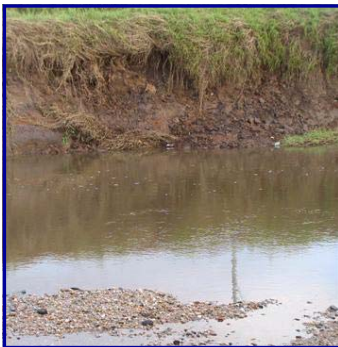
Severe bank damage counter-balanced by gravel deposits. (R S-W)
